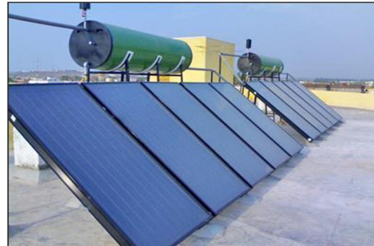
Flat plate thermal system for water heating deployed on a flat roof.
